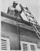
JACOBO FIGARAO , carpenter first class with over 20 years' service, starts the cut through the roof of a classroom to be moved to Santa Cruz.
